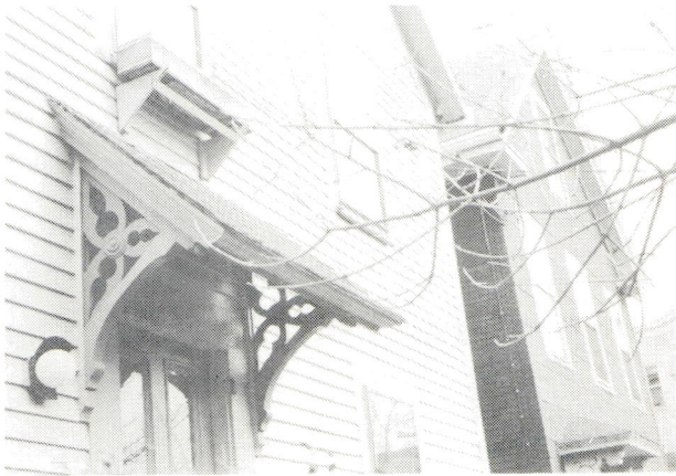
D23. "Tracery" holding up a sloping roof
