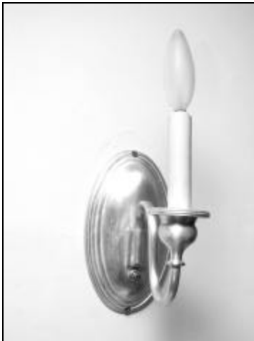
This sconce is one of many fixtures that needs rewiring. They were installed by the preservation architect Joseph Everett Chandler in 1916.
